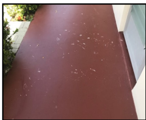
Carelessly splattered paint
